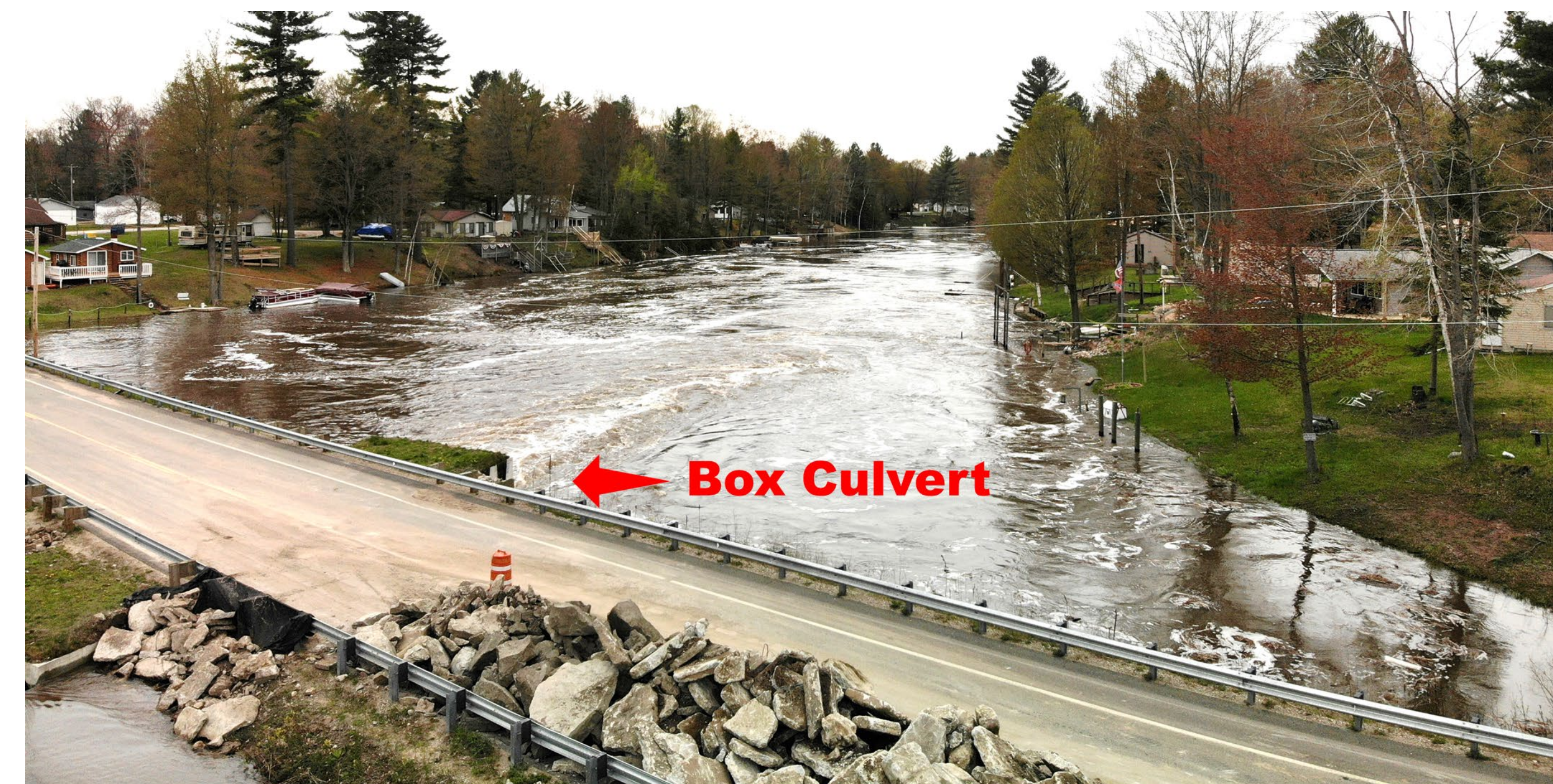
Stone was quickly brought in to stabilize the road and allow water to only flow through the precast concrete box culvert into Secord Lake.
