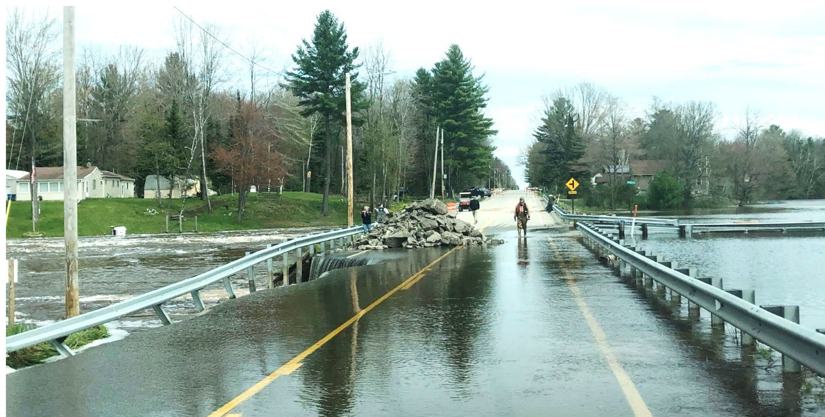
Gladwin County, MI, Wildwood Road (bermed roadway) was compromised during a 500-year flood event in May 2020.
