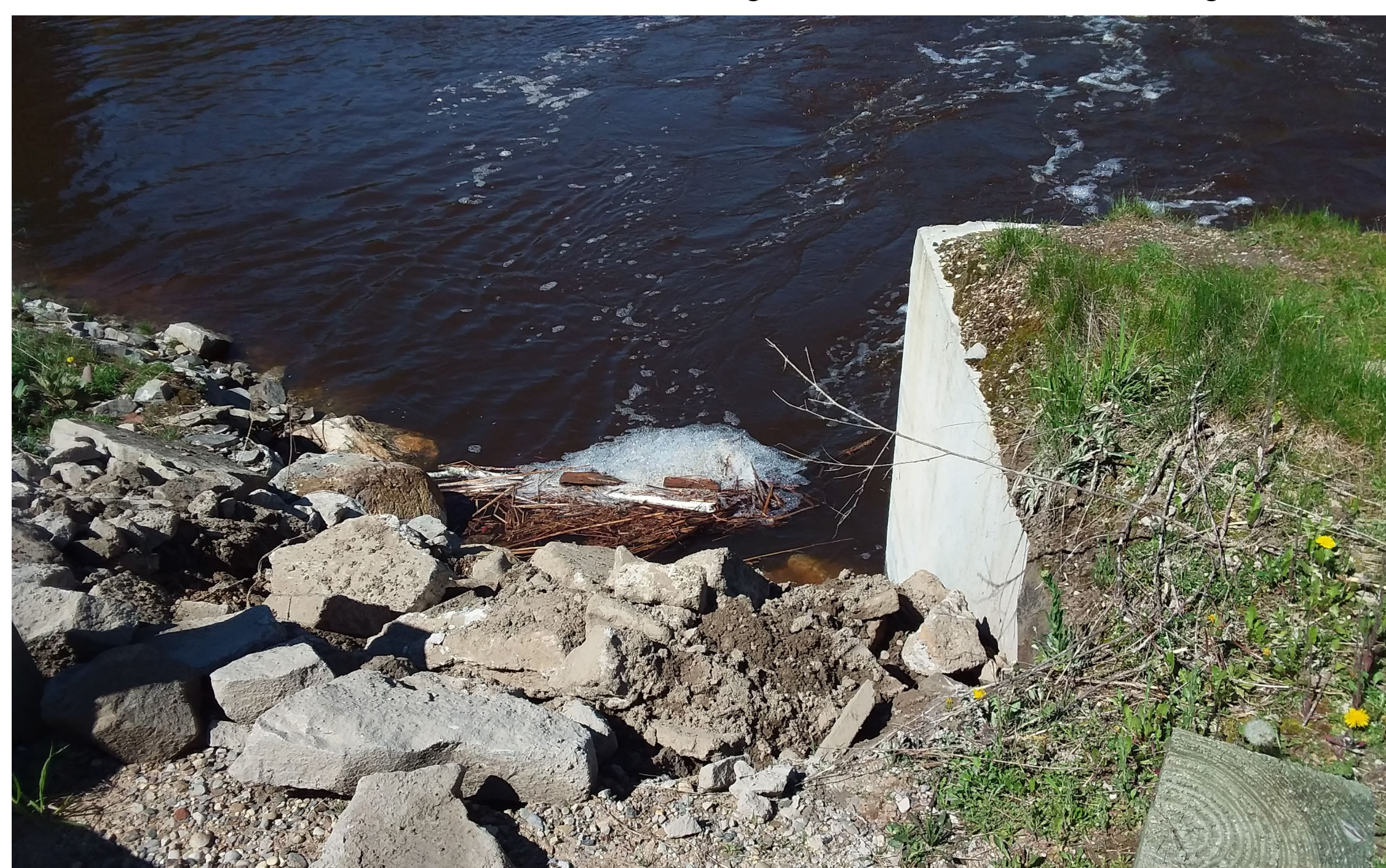
The Weight and Strength of the Precast Concrete Box Culvert kept Wildwood Road in place and prevented further flooding.
