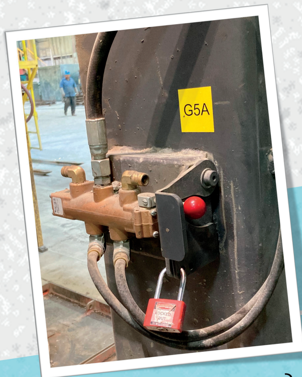
{Lock Out Point}
