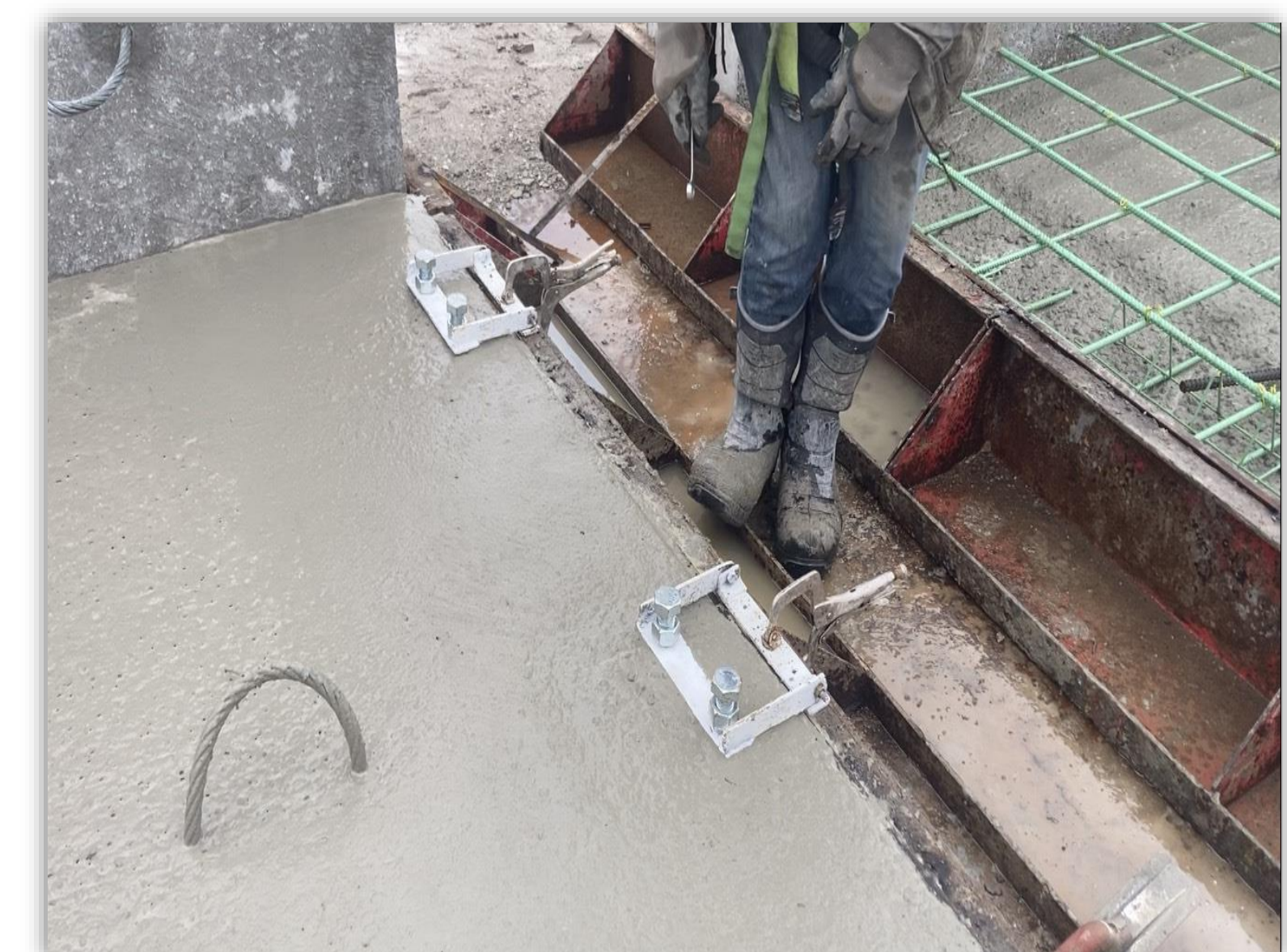
Once concrete is poured and finished, the anchor is dropped back into place and secured to prevent the anchor from shifting or sinking into the concrete before initial set.
