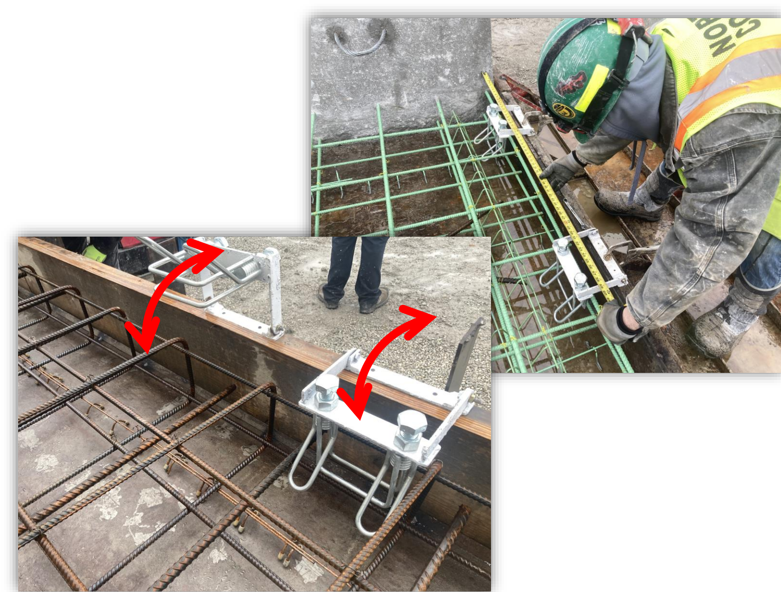
Drop-in anchor mounts are attached to the form where they are required, allowing QC personnel to do their pre-pour inspection and verify placement. This verification is required as part of the ACPA QCast program.
