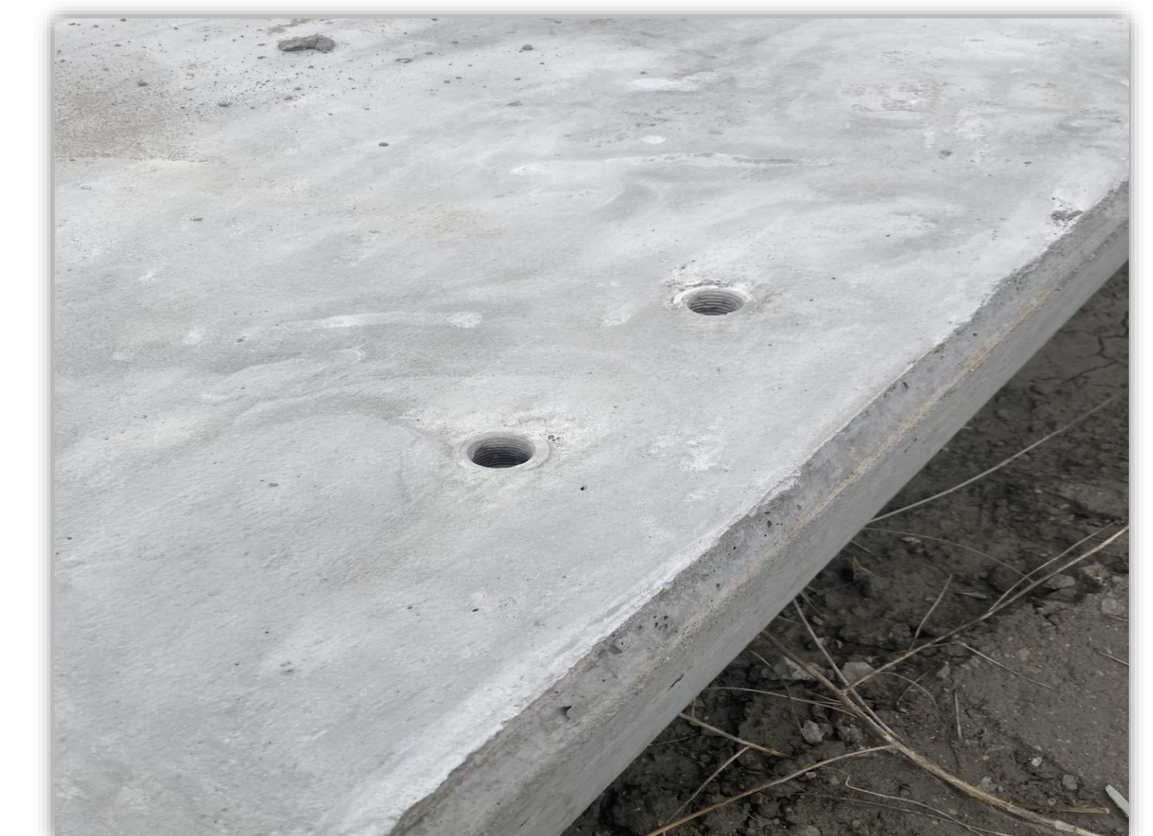
Using this method, we are guaranteed to get a neat, accurately placed, flush, and straight anchor every time!
